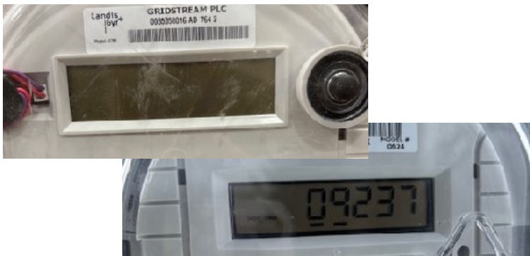
Pictured are a blank meter (top) and an operational meter receiving power (bottom)
