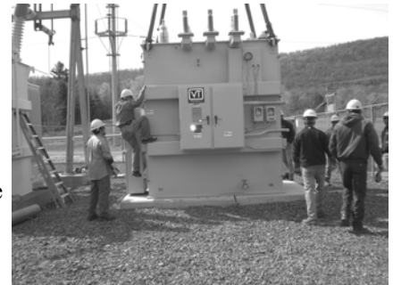
New Kortright transformer
