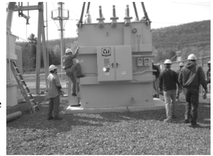
New Kortright transformer
