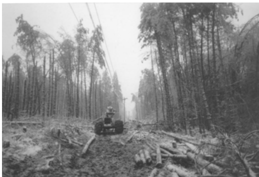
DCEC crews clearing downed trees from ice storm
