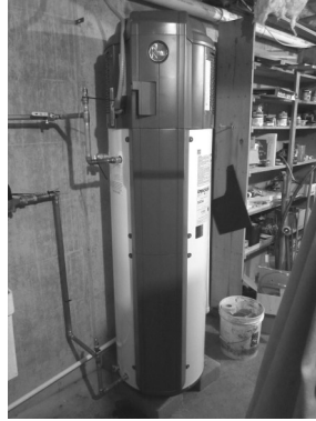
Heat pump hot water heater installed at DCEC member Tom Little's house
