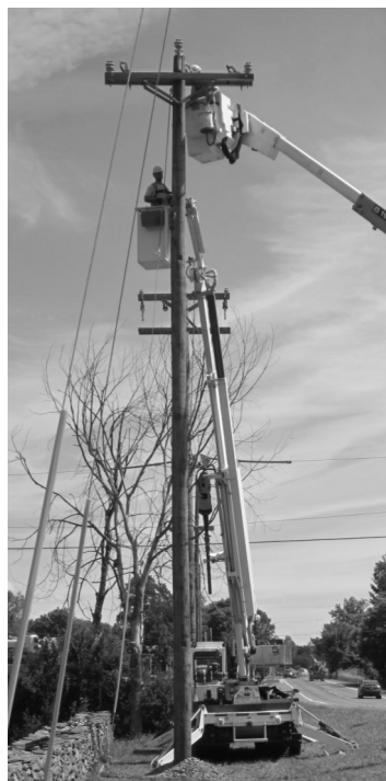
DCEC Linemen working on the interconnection with NYSEG on Route 23 near Zimmerman Road in Harperfield
